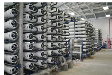
CSID's Nano-Filtration Water Plant
